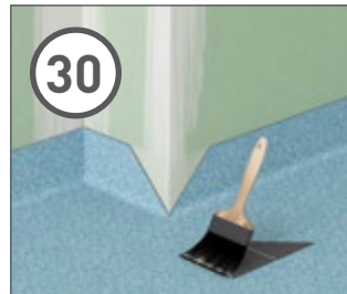
30 Use offcuts to fill in external corners, use heat to soften the vinyl so that it is easy to form tightly around the corner.
