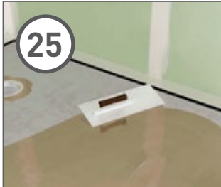
25 With a metal trowel, spread the adhesive onto the floor and coving, use a smaller spatula to apply adhesive round the drain hole.
