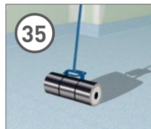
35 Roll with a 68kg articulated floor roller, firstly in the short direction, then in the long. In corners and other awkward areas, use a hand roller. Ensure that all the sheets are adhered.
