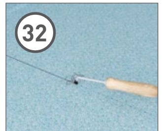
32 Use a grooving tool to groove all joints in the flooring before welding.
