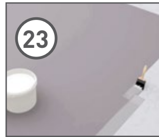
23 Lay the sheet face down and coat the edges that will sit on the coving with pre-mixed reactive adhesive.
